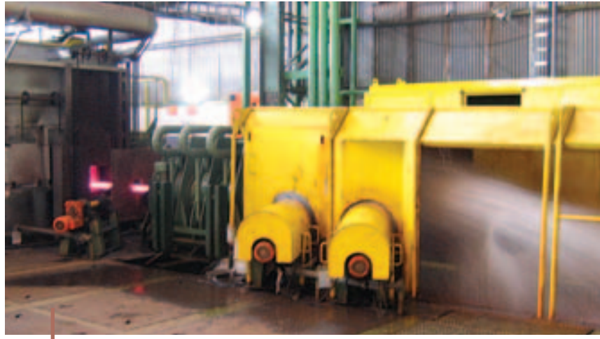
New tubing quenching unit
