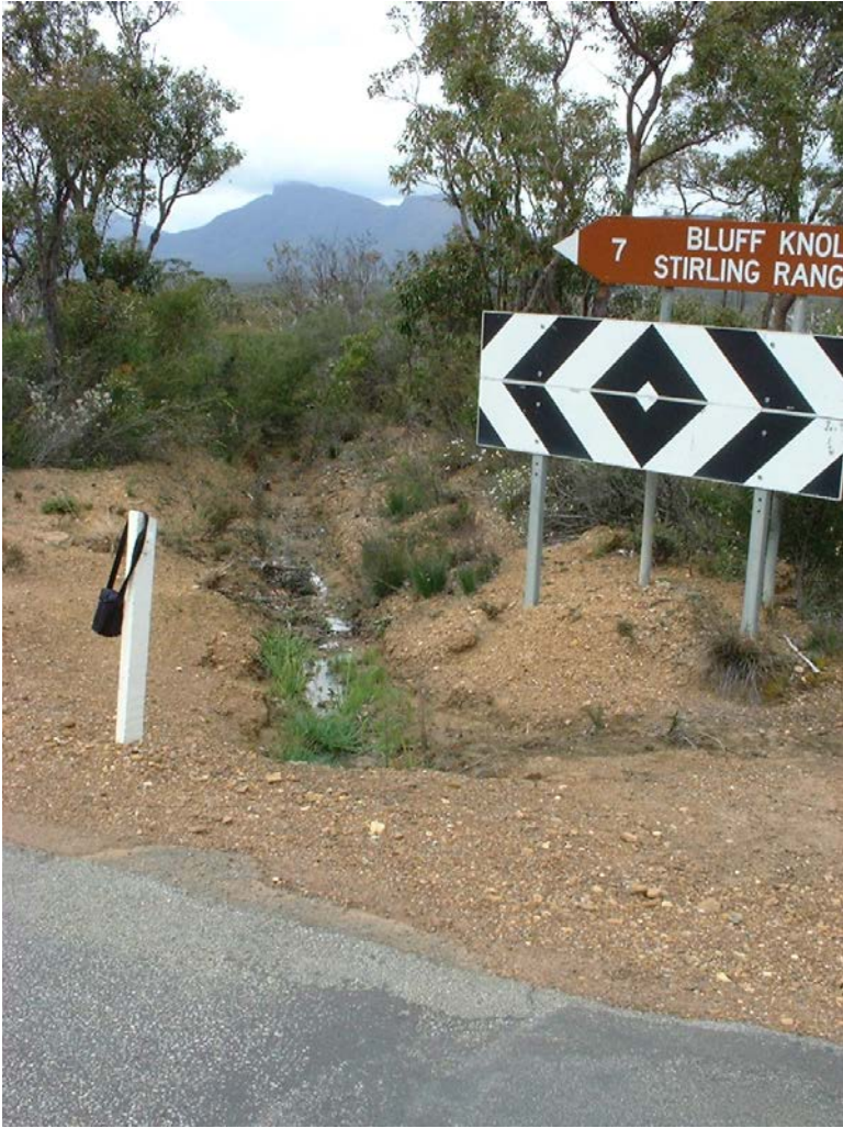
PLATE 6 – Culvert outlet drain to diagonal skewed culvert at junction of intersection on eastern side
