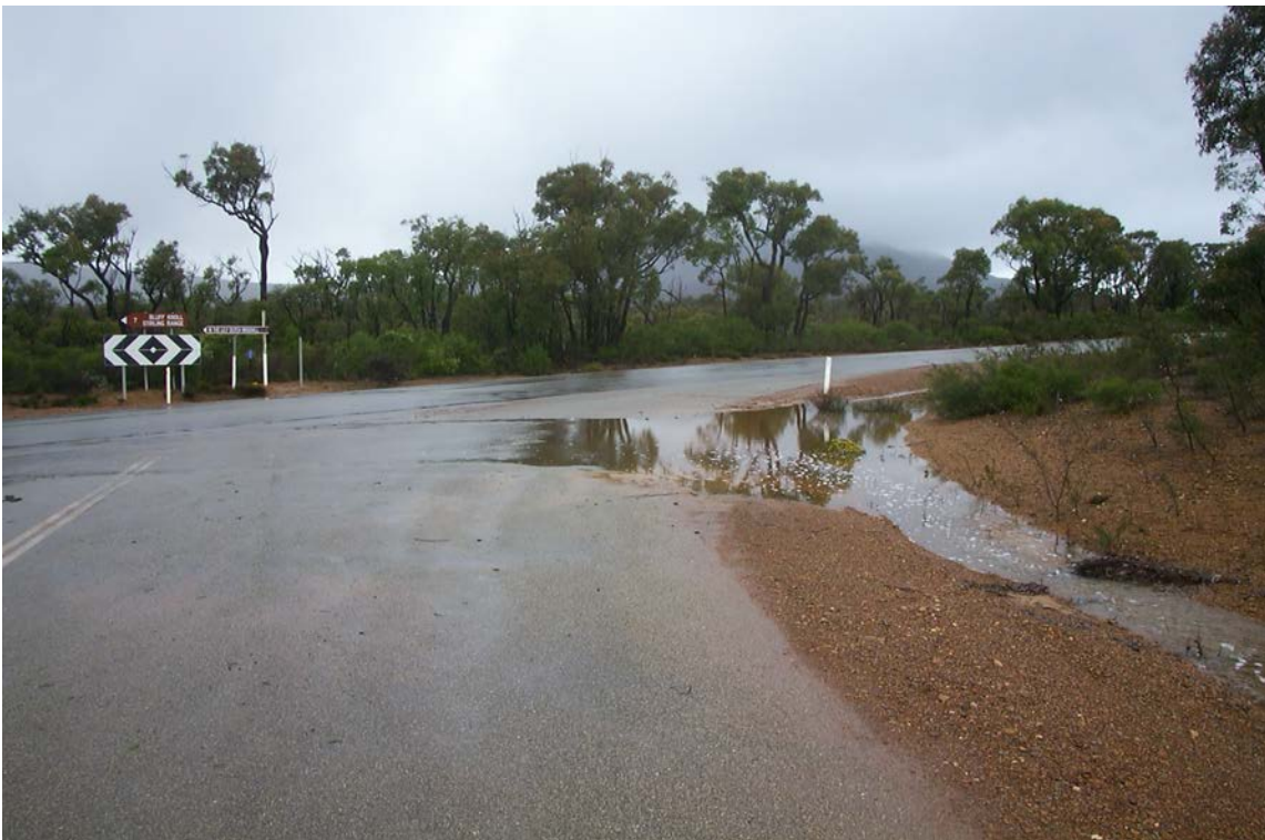
PLATE 11 & 12 Photos taken previously on 1 October 2003 showing extent of flooding on the southern side of Formby South Road at the Albany – Lake Grace Road intersection. Culverts to be upgraded (increased in size) to accommodate this excess water without changing drainage pattern.
