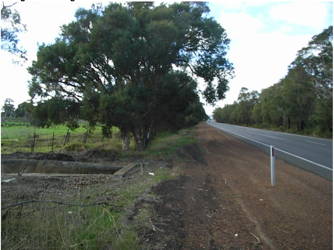
Photo 9: SLK 143.0 View north east showing culvert and irrigation drain crossing under the road – clearing on left side
