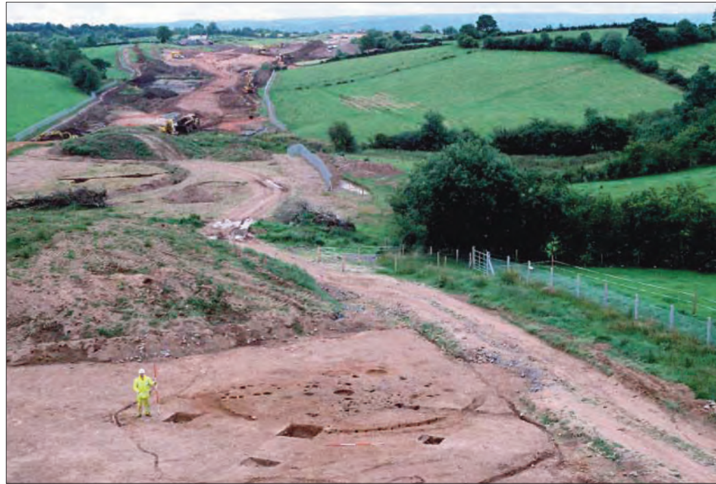
House site at Golan (Site 28) with road being constructed to back of photo © ADS
