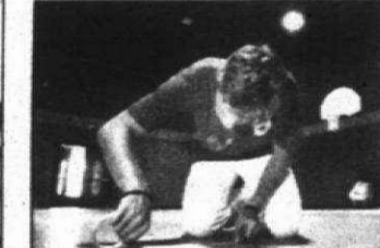
Jamie McEntee puts masking tape on the Hoben gym floor in preparation for a paint job.
