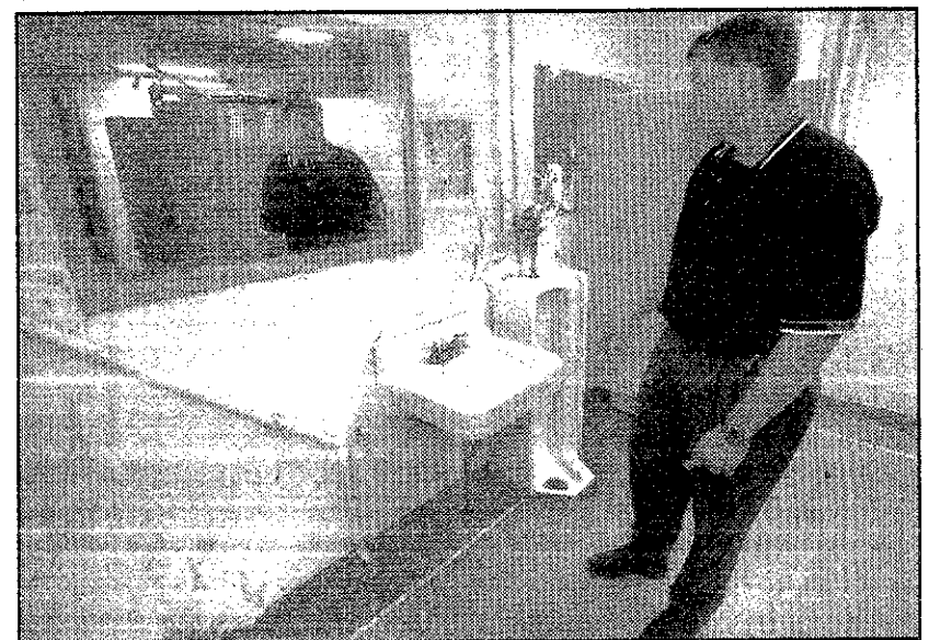
Bathroom problems: Teacher and football coach Ernie Crumm shows that the sink and toilet facilities are in poor shape in the football locker room. Rust-colored water runs from this faucet and others in the building.
