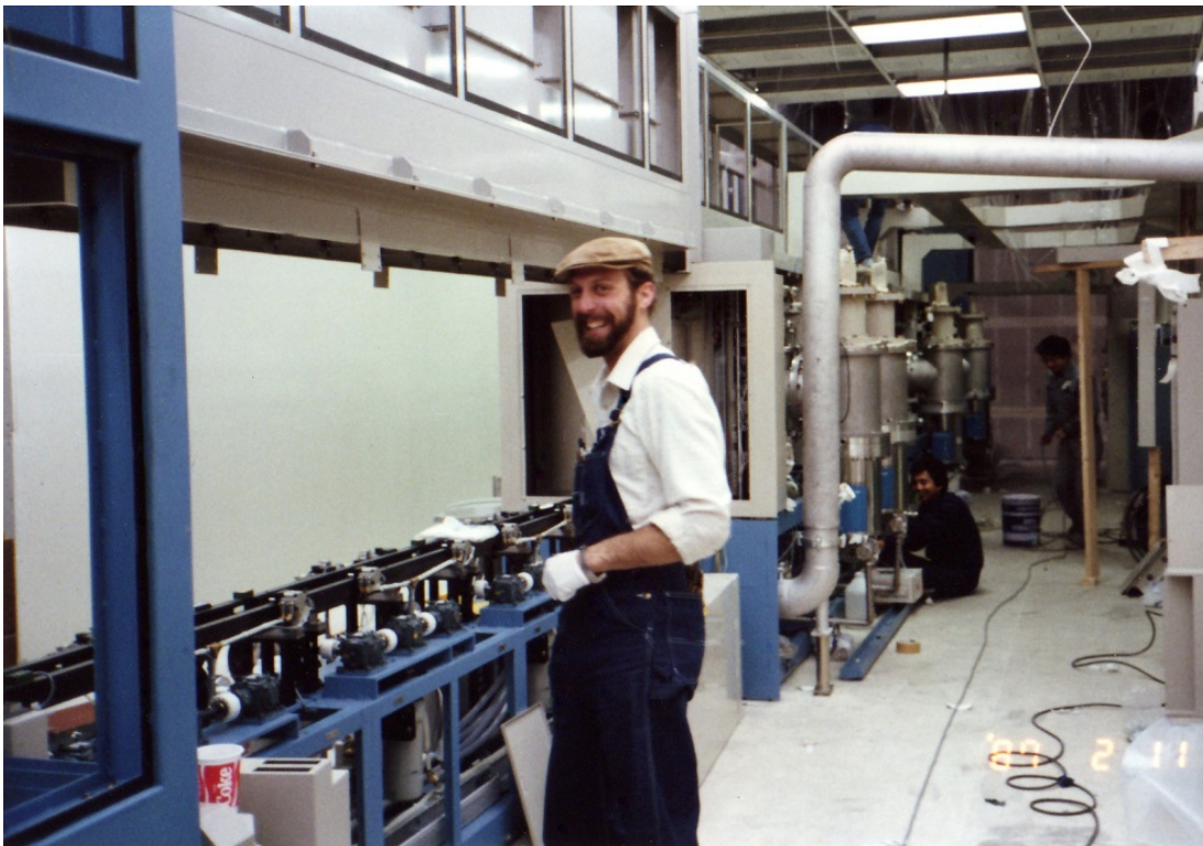
Sputter system under installation in Bldg. 2 of the S. Hillview facility. The engineer is Dan Levien, one of Ron Allen's guys. The ULVAC installation team is in the background.
