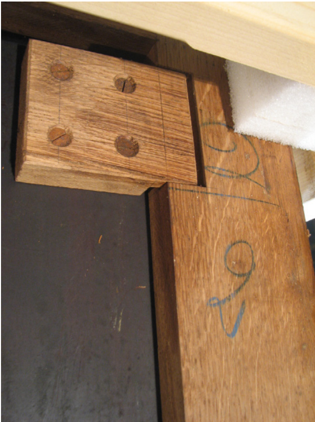
Fig. 5. Slip joint with French witness marks on the cradle
