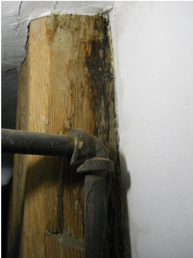
Fig. 2. Dark-colored staining on historic oak post, pew 38 area, 2015 (Courtesy of the author)
