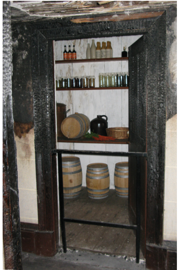
Fig. 3. Example of the extensive damage to millwork caused by the fire (Courtesy of Deborah Hudson)
