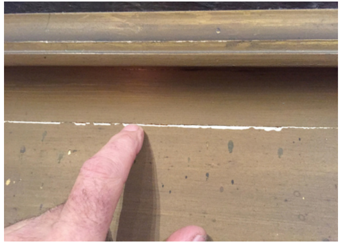
Fig. 3. The joint line along the two large frame members was failing and especially visible along the bottom rail.
