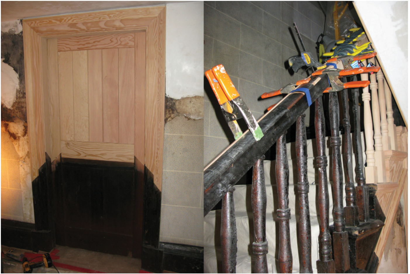
Fig. 10. Replacement millwork surrounding the entrance to the larder (a) and replacement spindles and handrail components installed in the balustrade before finishing (b) (Courtesy of Deborah Hudson)
