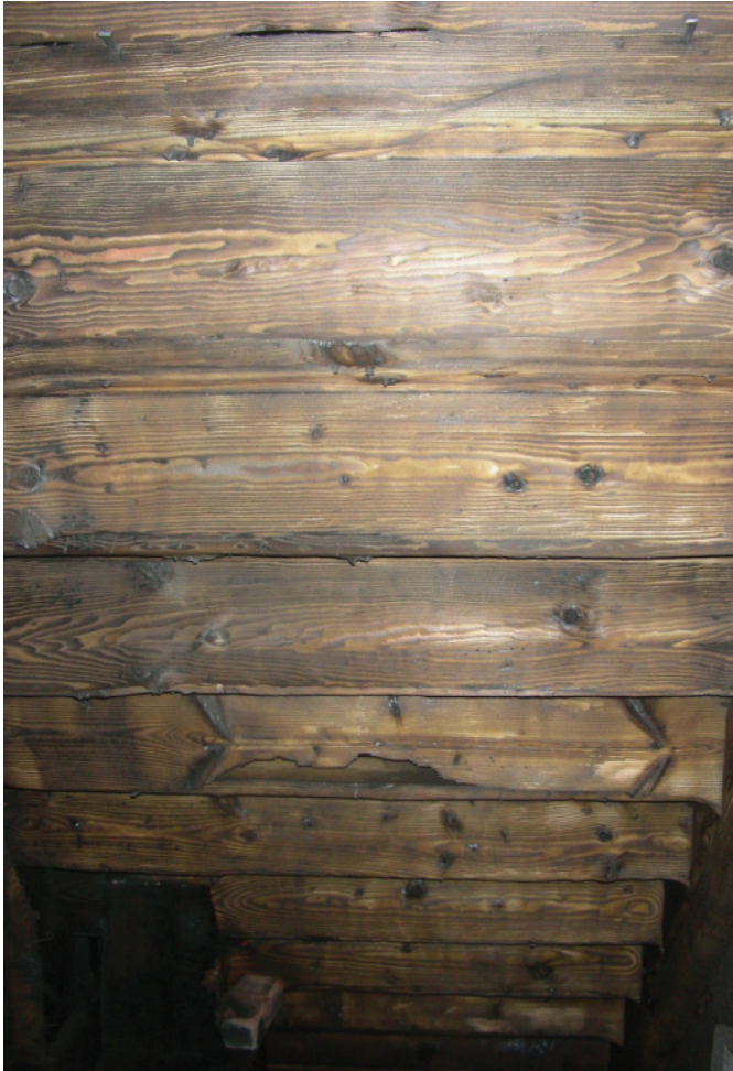
Fig. 8. Staircase substructure after dry ice blasting treatment (© Government of Canada, Canadian Conservation Institute. CCI 100841-0053)
