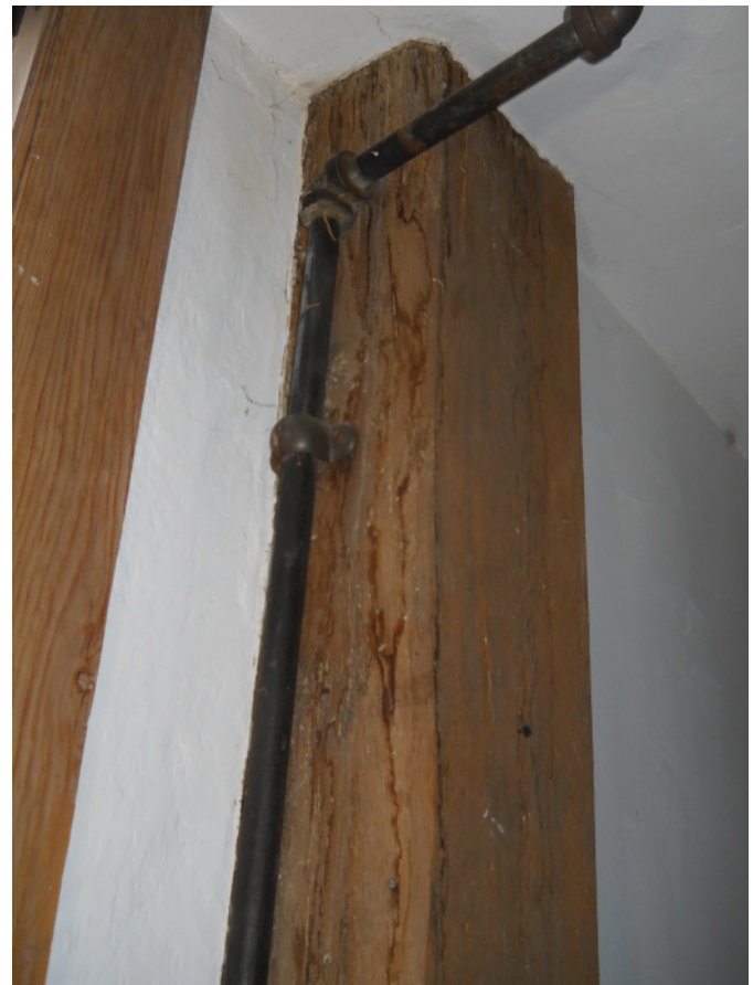
Fig. 3. Ferrous metal sprinkler pipe and head (ca. 1930), contributing to adjacent wood waterborne staining, 2015 (Courtesy of the author)
