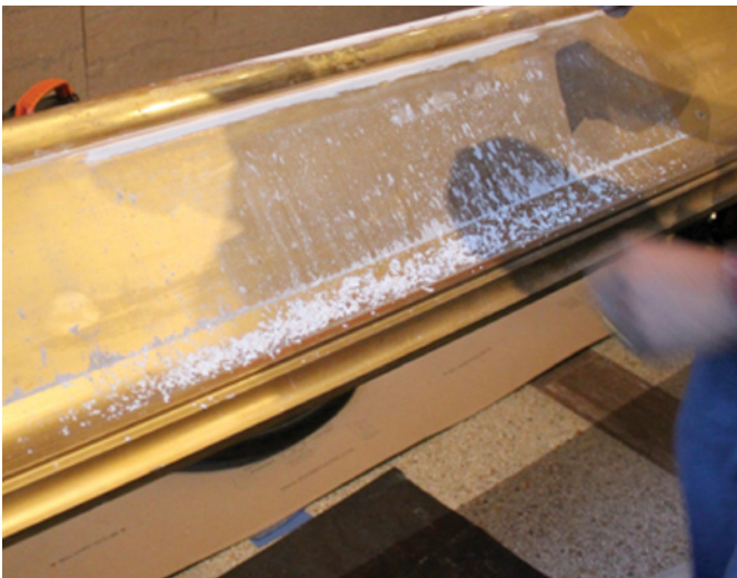
Fig. 14. Cracking and areas of loss along the frame were filled with putty and sanded down to match the existing contours of the frame.
