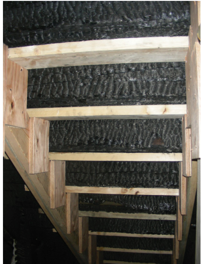
Fig. 6. The auxiliary support installed to support the damaged staircase (© Government of Canada, Canadian Conservation Institute. CCI 100841-0025)
