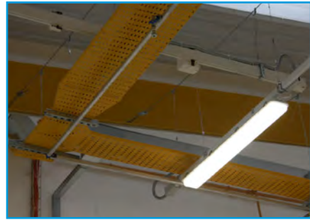
Busbar and Lighting
