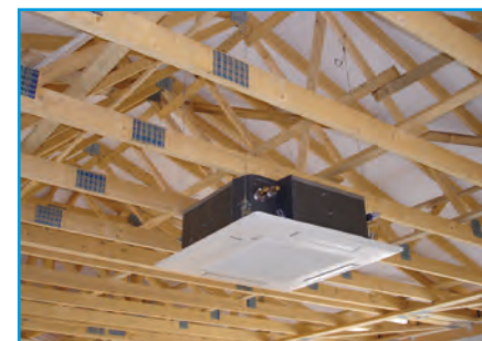
Air conditioning units
