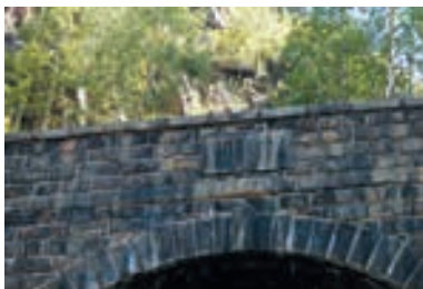
← A tunnel arch on the Circum-Baikal Railway Line in the vicinity of Cape Tolsty
