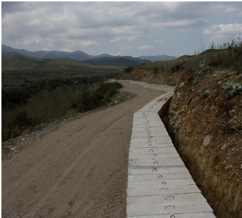
Photo 69. Newly constructed irrigation system which intersects with the route of highway alignment B (near village Miravci).
