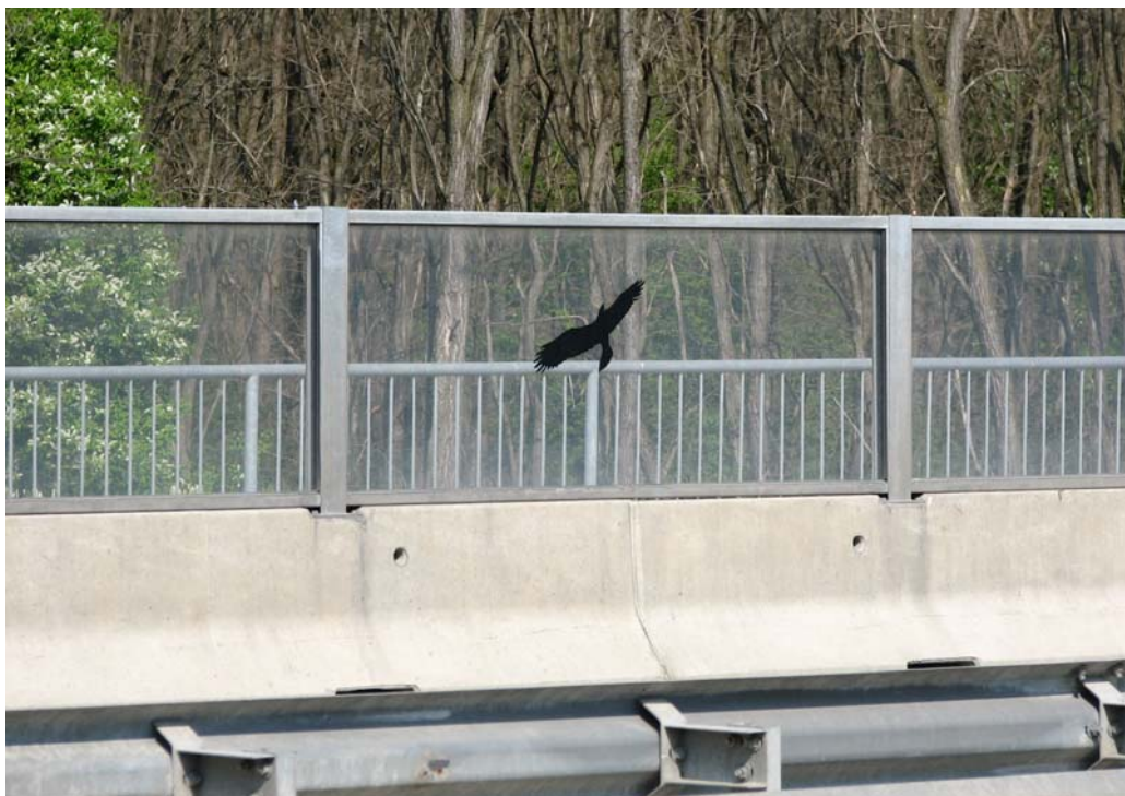
Photo 74. Detail of the protective panels for prevention of bird kills
