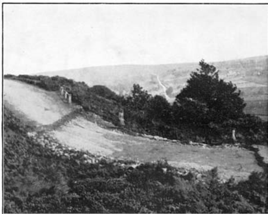
COUMS. SINKING OF ROAD AFTER FLOODS OF SEPT., 1931.
