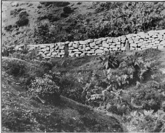
COUMS. ILLUSTRATING SINKING OF ROAD.
