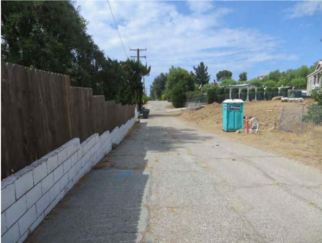
Photograph 5: View of the proposed pipeline location along Apple Tree Lane in the northern portion of the Apple Tree Lane Survey Area, facing southwest.
