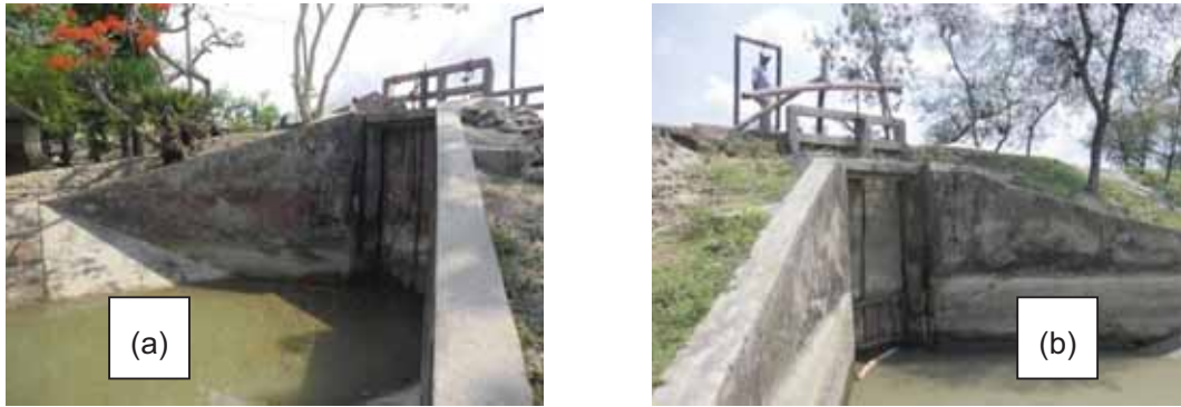
Photo 4.3: Drainage Sluice at (a) Katia Nangla Khal which needs replacement of gate and railing, (b) Moisher Danga khal which needs similar replacements
