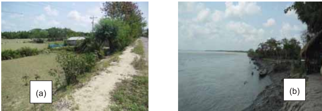
Photo 4.2: Existing Status of Embankments(a) Narrow earthen surface along the peripheral embankment (b) Erosion point at Sholmari with nominal setback distance)
