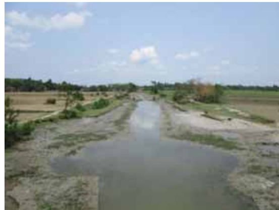
b. Kalatola Khal (Silted Up)
