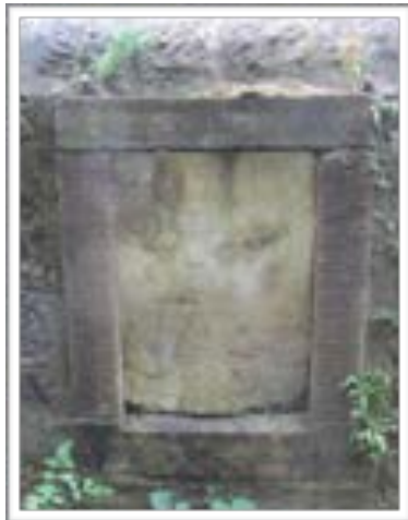
Inscription panel missing
