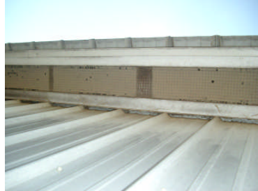
Sofits blocked with dust
