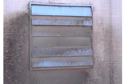
Fan louvers shut with dirt
