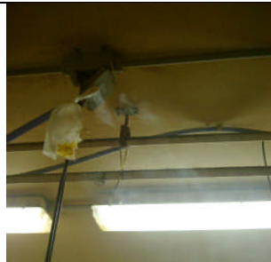
Lights diverting air patterns
