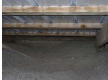
Insulation blocking soffit
