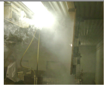
Power board obstructing air flow
