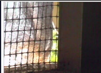
Poor curtain maintenance
