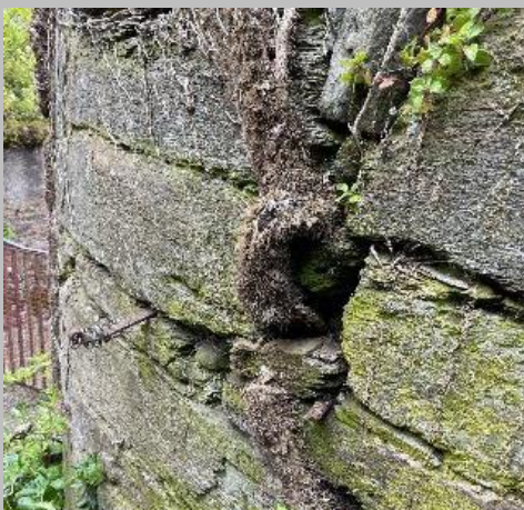
Embedded ivy roots at tower base
