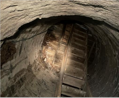
Timber decay in third floor and suspended timber stair
