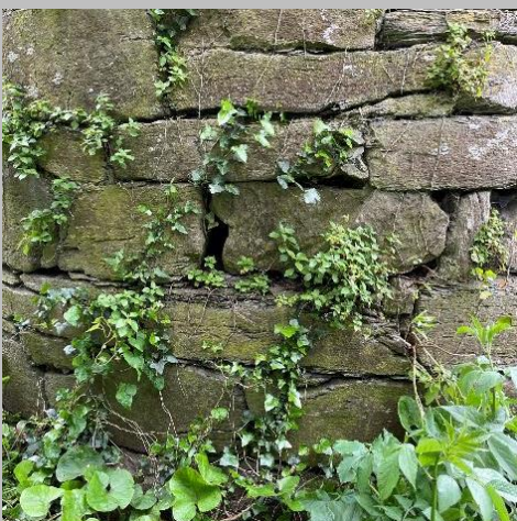
Bed joints fully eroded – stones bearing directly on each-other
