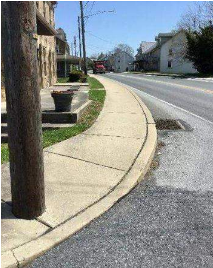
Sidewalk Obstruction - Utility Pole
