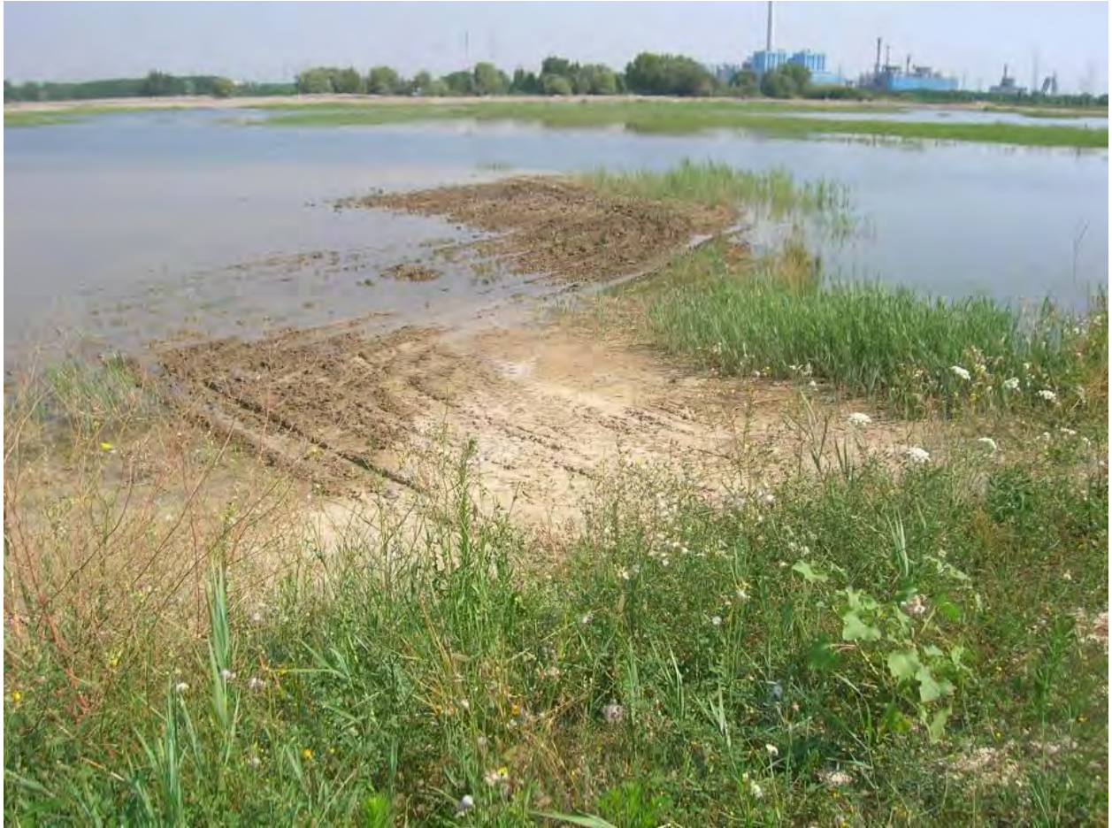
Figure 6.1: Uneven grading and machinery marks left during grading of a constructed treatment wetland.
