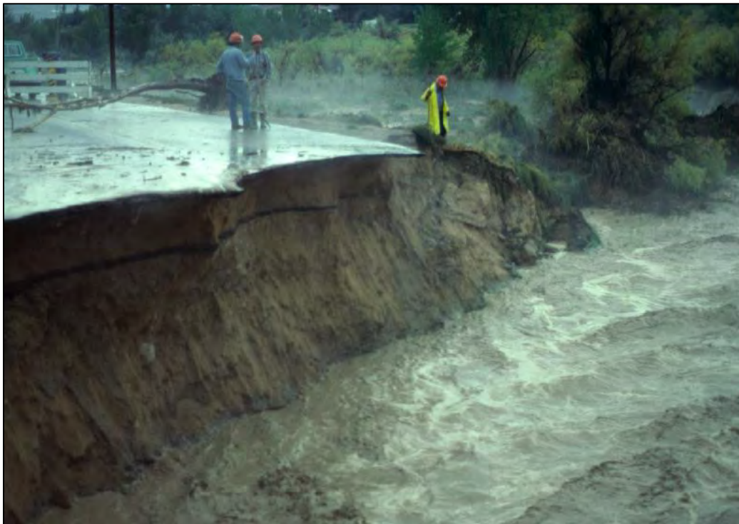
Photo 41. Wash-out along Monument Road on 7 September 1978 (Photo by Jim Johnson, from Richard 2004).
