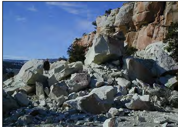
Photo 39. Rock fall onto Rim Rock Drive in January 2000 (NPS photo by Ron Young).
