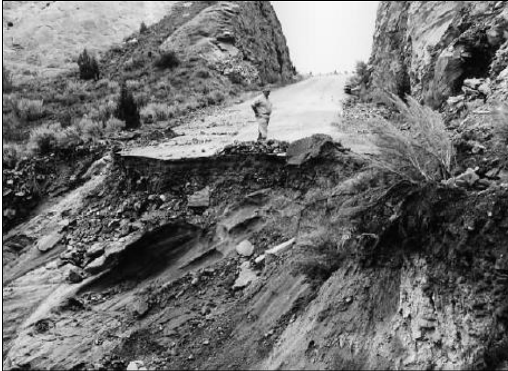
Photo 40. Section of Rim Rock Drive washed out by flooding above the west entrance in August 1968 (NPS photo).
