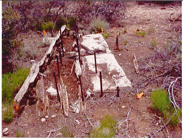
8. Mill foundations located on the west side of the main mining pit.
