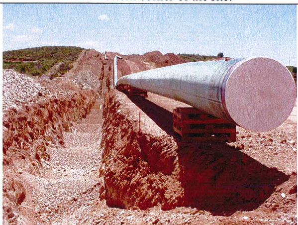
12. New gas pipeline being installed across the southwestern corner of the site.
