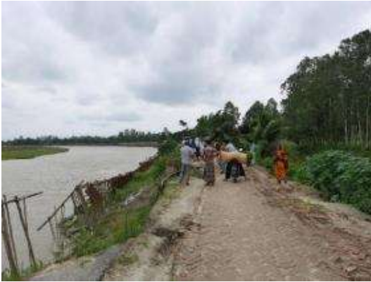
Fragile road network along the riverside
