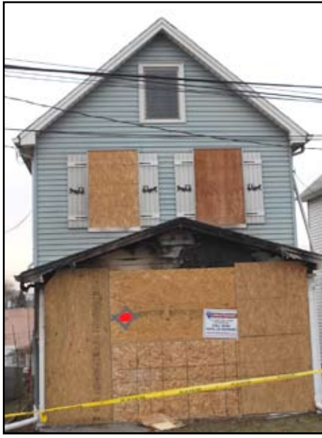
This Catherine St. home in South Amboy is boarded up after being severely damaged by an early February fire. (Photo by Tom Burkard)
