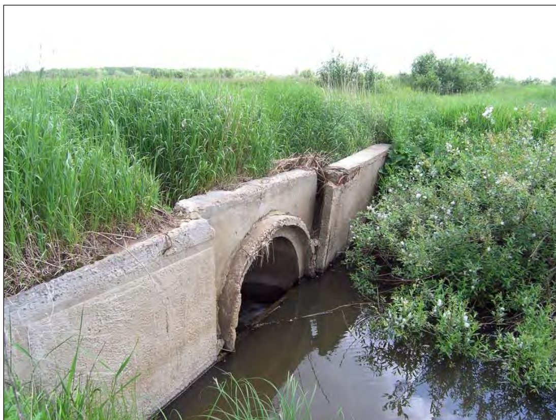
Photo 2. A wooden shield in a concrete pipe under the crossing between the fields, June 2002 (photo by O.S. Grinchenko).
