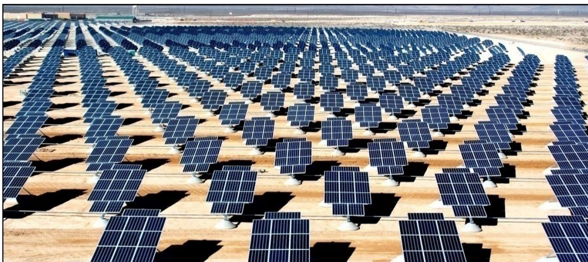
Fig. (II.22) Photo illustrant un champ photovoltaïque
