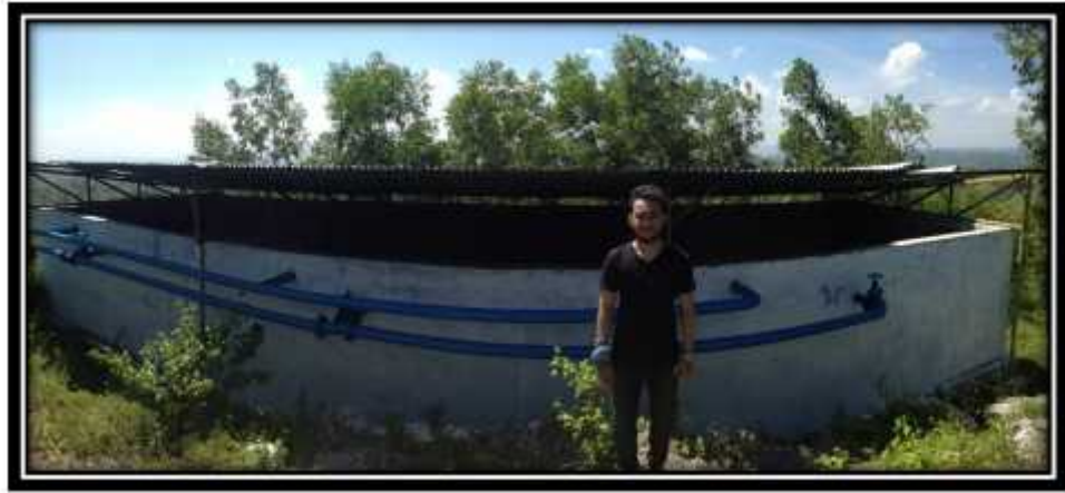
Gambar 4.5. Instalasi Pengolahan Air Saringan Pasir Lambat Kaligoro (x=464818; y= 9109887)
