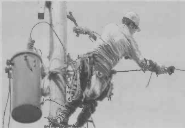
A ComEd crew lineman works high on an electric pole to restore power last summer. | KEITH HALE-Sun-Times Media
