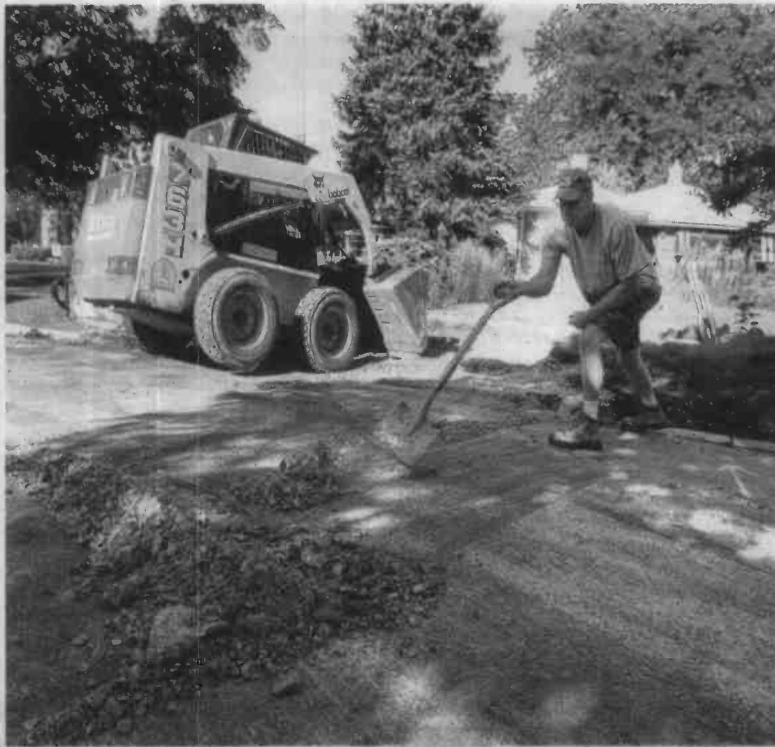
Park Ridge Public Works employee Pat Navin shovels debris during a water main break restoration in August. Dry summer weather has been blamed for an increase in main breaks this year. | BUZZ ORR-Sun-Times Media
