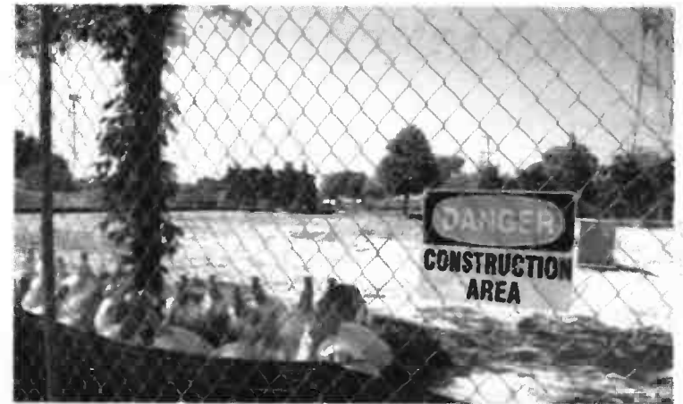
Oriole Pool, located at 9200 Oriole Ave., has been demolished and the park district has been given permission to start construction on a new facility in September. | RICK KAMBIC-Sun-Times Media
