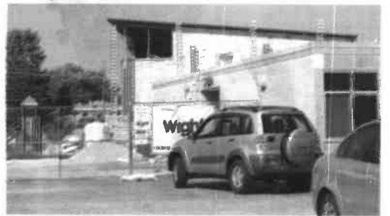
District 67's new 6,400-square-foot gymnasium outside Hynes Elementary School is scheduled to open in January. It's the main unfinished component of the renovation. | RICK KAMBIC/SUN-TIMES MEDIA
