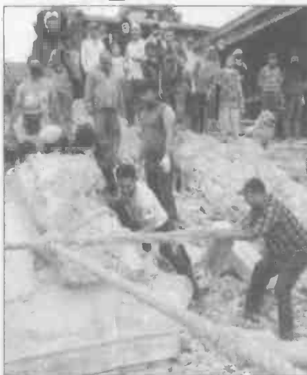
INTERNATIONAL FEDERATION OF RED CROSS PHOTO Nepalis help to remove rubble from the ancient Mahadev Mandir temple at Durbar Square in Bhaktapur, Nepal, April 30.
