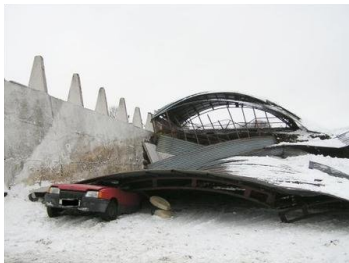
Fig. 1: Ruined hall roof.
