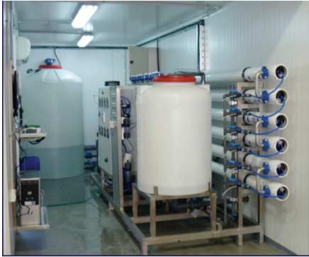
The first-generation desalination pilot plant.
