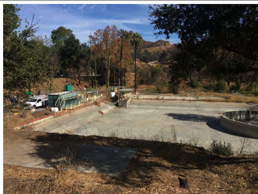
Photo Location 2. December 2019. View of permanent wastewater treatment plant site to the left with oxidation basin to the right.
