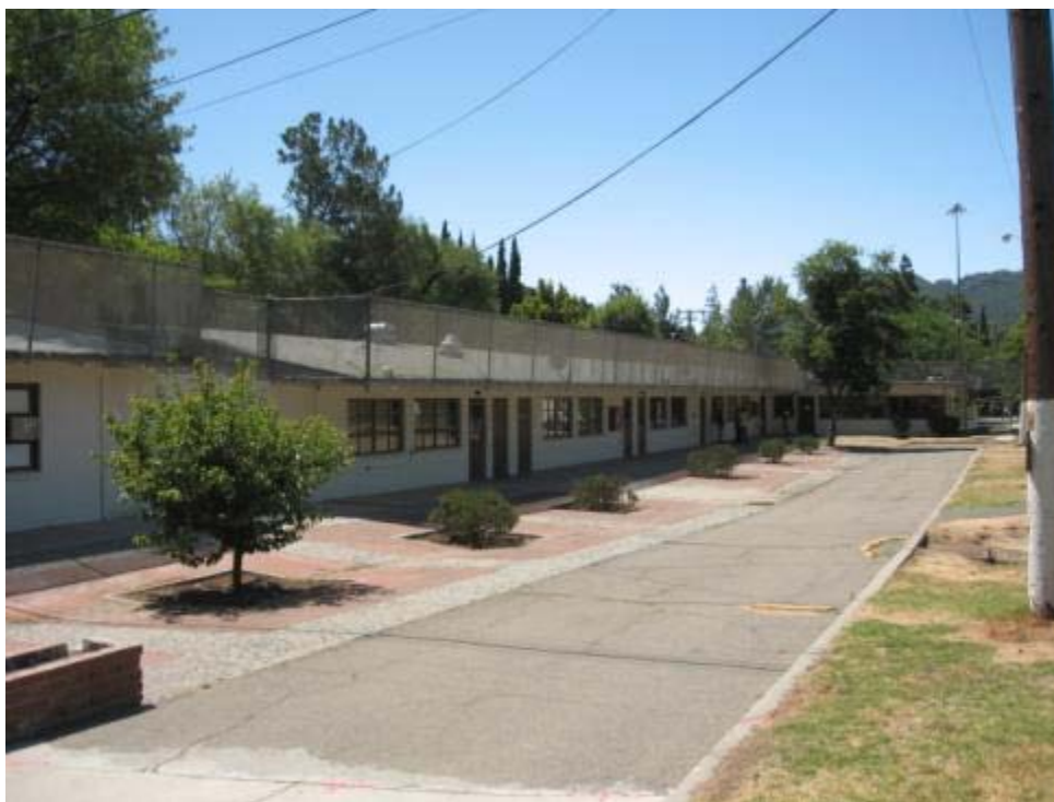
Classroom building and attached Principal's Office (at far end). View looking south.
