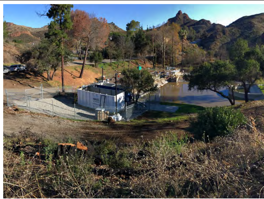
Photo Location 1. December 2019. Overview of project site with temporary wastewater treatment plant in foreground.
