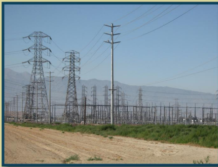
Mira Loma Substation
