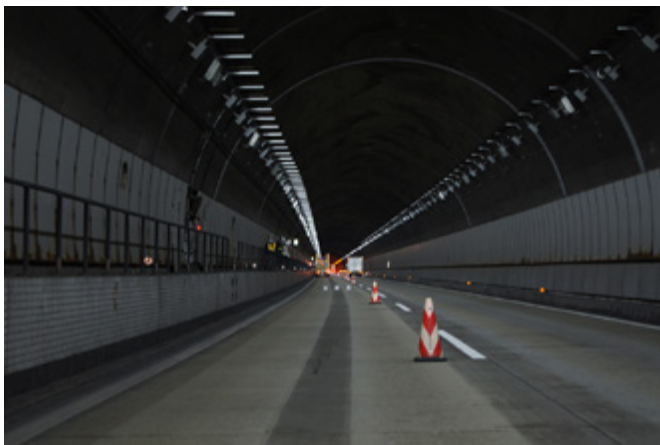
Figure 1 - Pro-beam lighting system
