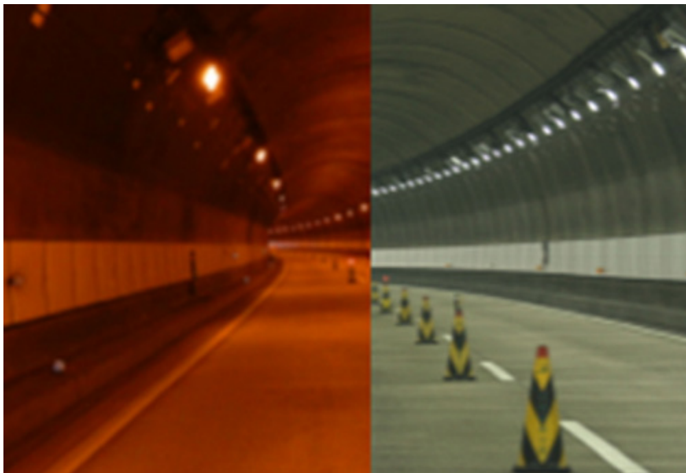
Figure 2 - Examples of tunnel installation (left: low uniformity, right: high uniformity)
