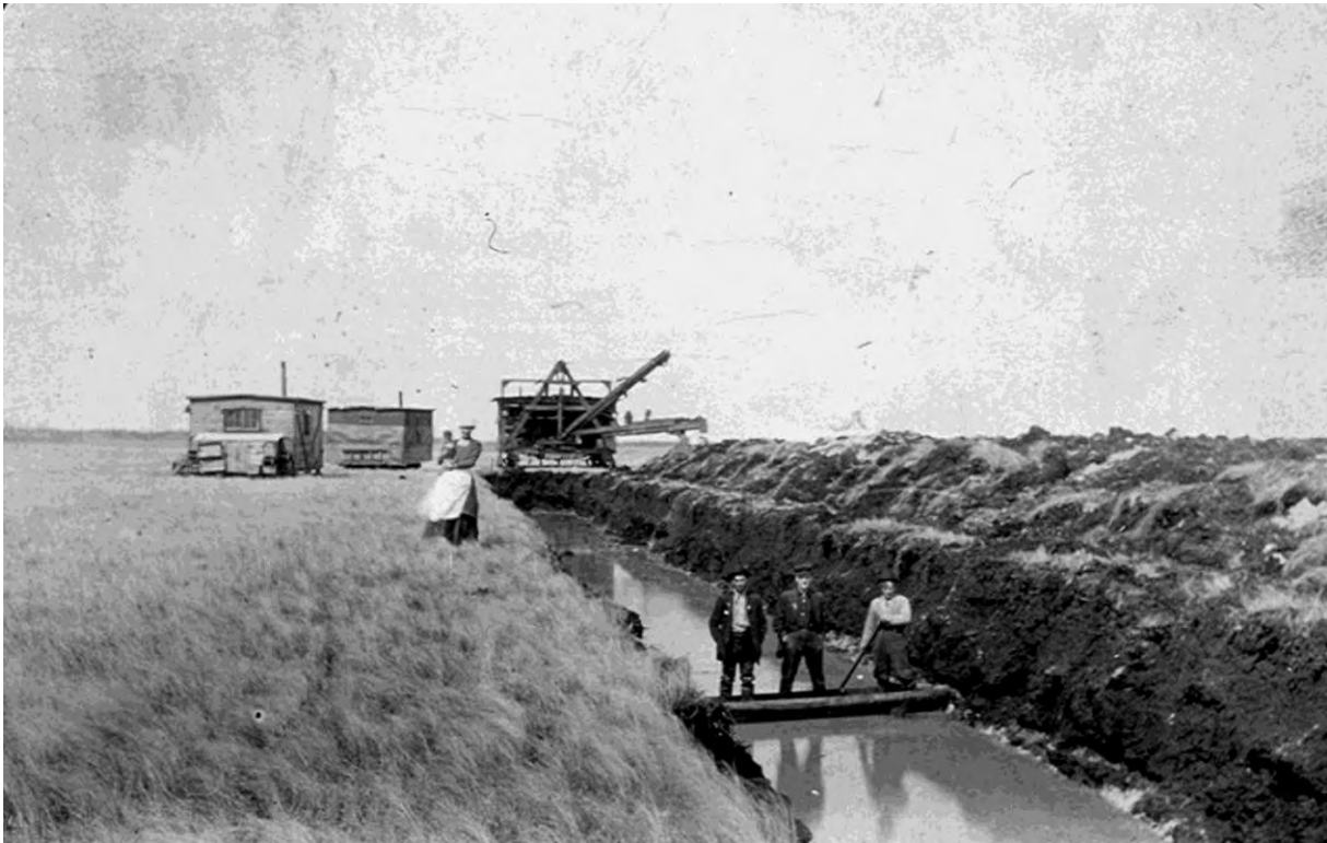
Figure 1.5. Ditch digging on the Joseph Dostal farm in Beltrami County, circa 1915. Photo courtesy of the Minnesota Historical Society.
