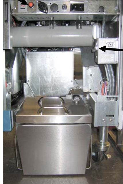
Melting unit power switch
