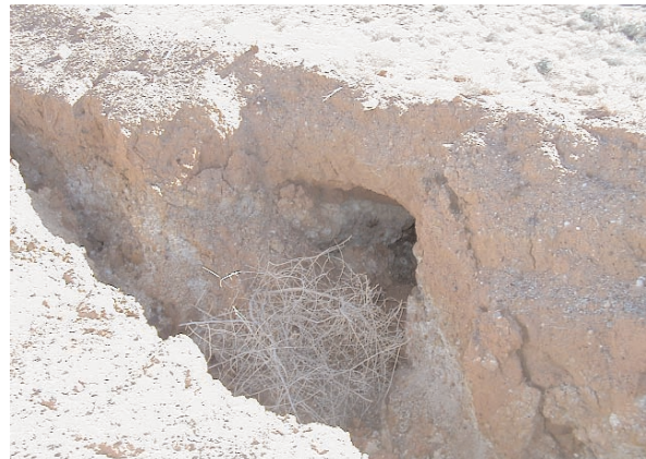
Figure 1: Tunnel developed from a berm on a waste rock dump constructed of sodic spoil.
