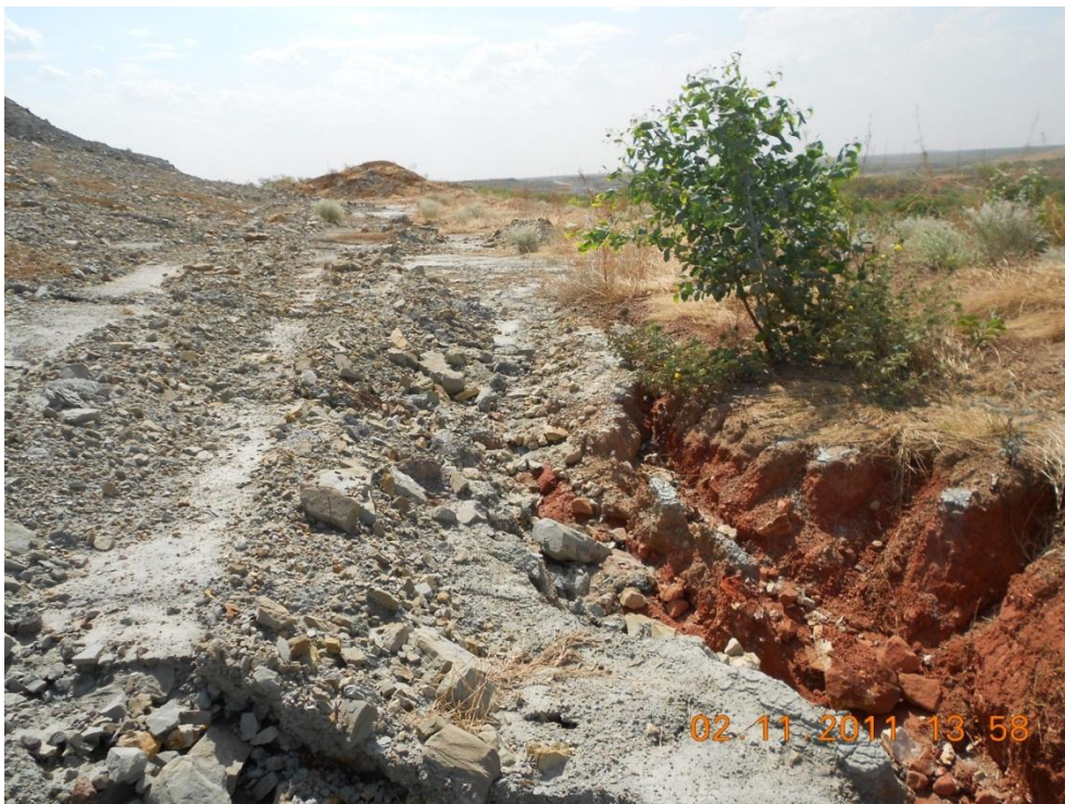
Figure 2. A sloping section of berm that is concentrating flow laterally to a point where it has overtopped and created a large gully feature on the batter below.
