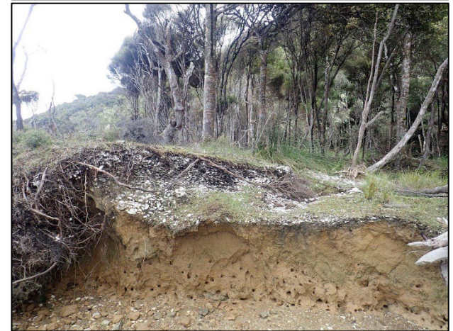
Bank erosion on north side of estuary west arm.
