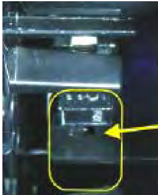
Incorrect alignment—gap between sensor and flag
