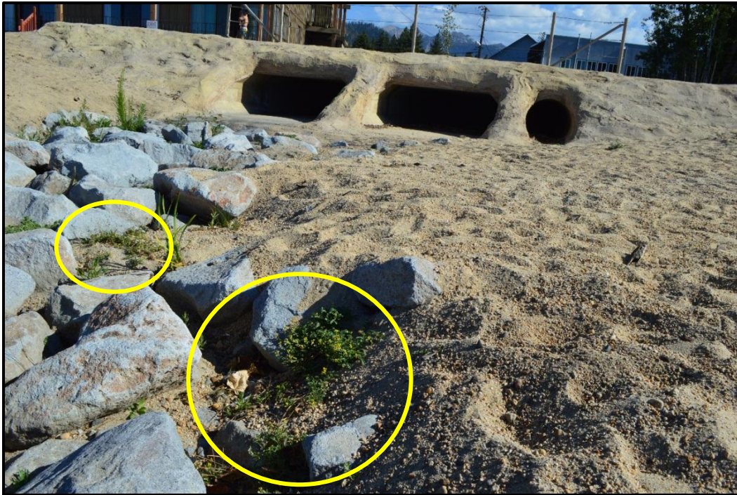
Figure 3.3. TYC growing among the rocks in September 2014 in the outfall constructed for the Bijou Area Erosion Control Project in South Lake Tahoe, California.
