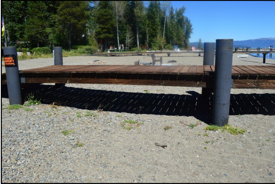
Figure 3.2. TYC growing around pier footings at Blackwood Beach in Placer County, California, in September 2014.
