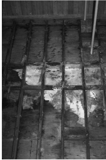
Fig. 8.8. Decay fungi growing inside the wall of a gymnasium. During construction, the wall's interior moisture barrier was intentionally torn, allowing moisture to intrude. Decay was apparent after removal of the wall panels. (Photo courtesy of Dr. Edson Setliff, Adjunct Professor, State University of New York College of Environmental Science and Forestry, Syracuse, NY.)
