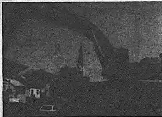
A rare sight on West Broadway, Hicksville indeed! St. Ignatius Church steeple is framed by the huge earth mover excavating a foundation for Ivan Czipott's eagerly-awaited small office building, north of West Marie St.
