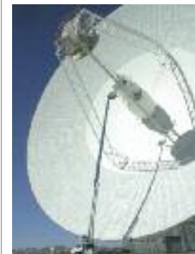
Scheduled maintenance for NASA's 70-meter antenna is performed by IBEW Local 543 members.
