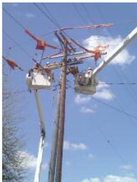
Local 51 journeyman linemen Jason Crabb and Ken Yokem are joined by apprentice linemen Joe Kindred and Jason Scott on a job for L.E. Myers, working under foreman Bill Steffey.
