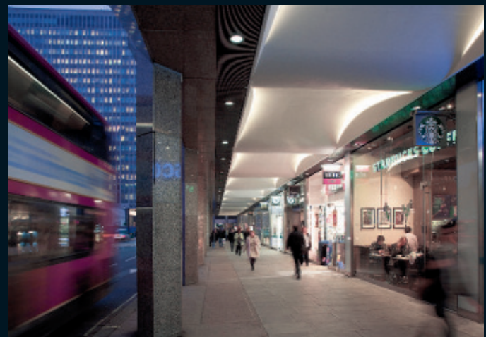
123 Victoria Street, lighting installation, London. Architecture: Aukett Fitzroy Robinson and Morey Smith.
