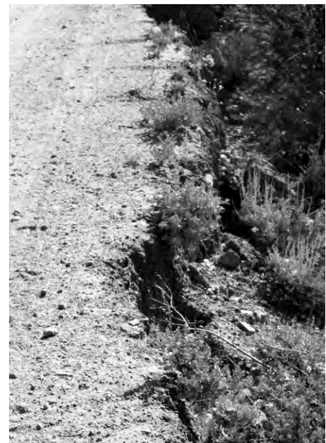
Figure 12: Swauger Road Erosion (Rick Kattelman)
