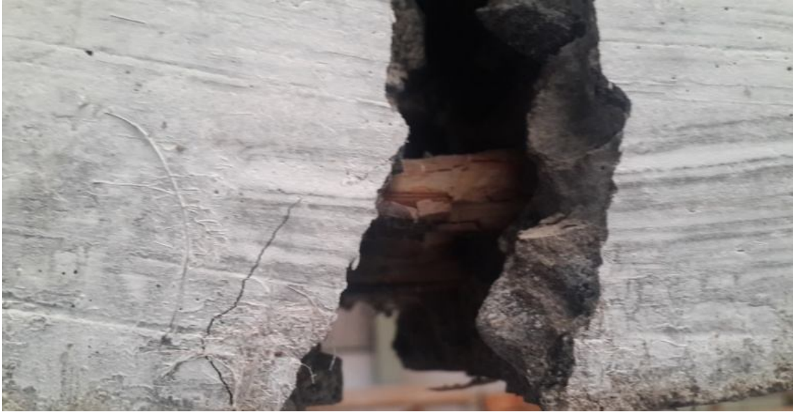
Plate 4.24: Slipped L. buchananii tensile reinforcement
