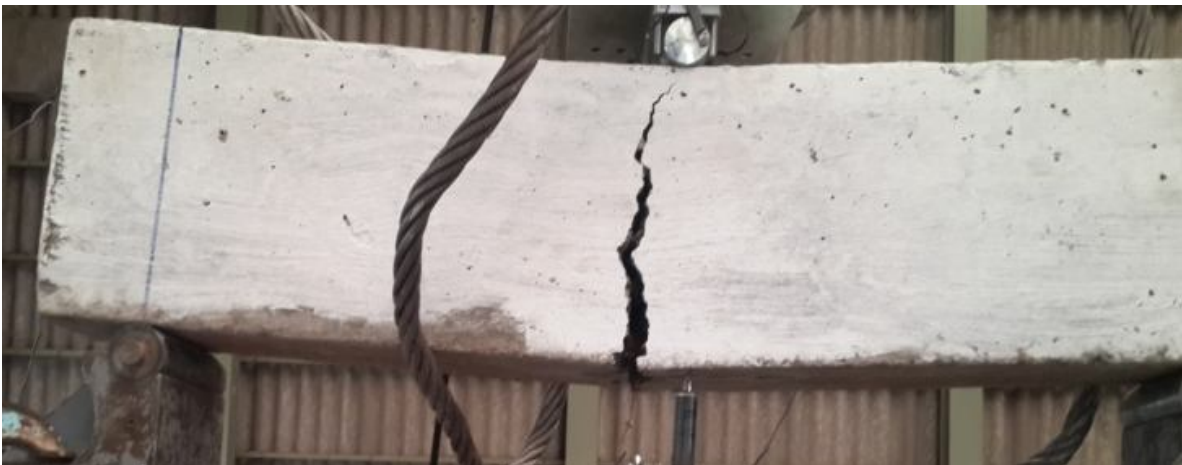
Plate 4.11: Failure pattern of L.B.399 beam
