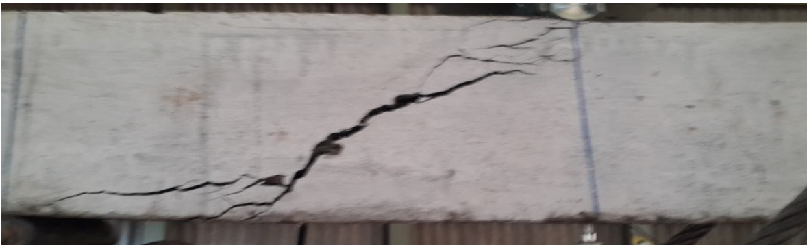
Plate 4.16: Failure pattern of L.B.1x8 beam
