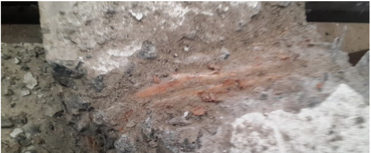
Plate 4.19: unbroken shear reinforcement for L.B.2x13 beam
