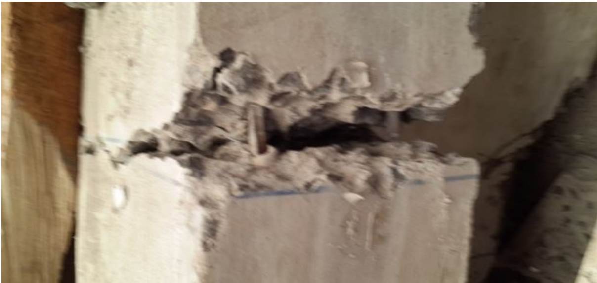
Plate 4.23: Snapped steel tensile reinforcement
