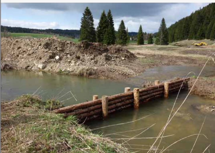
Figure 10. Drainage and blocking dam.
