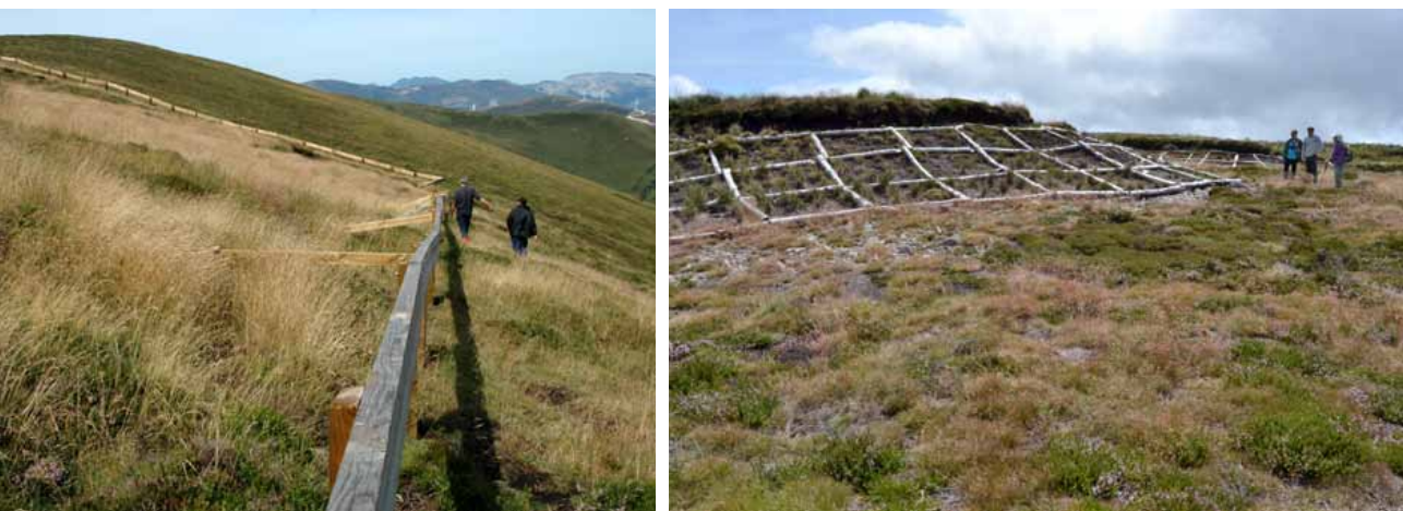
Figure 11. Restoration actions at the Zalama blanket bog. View of the protective fence in 2014 (left). View of the covering of the peat fronts with geotextile, also in 2014 (right).
